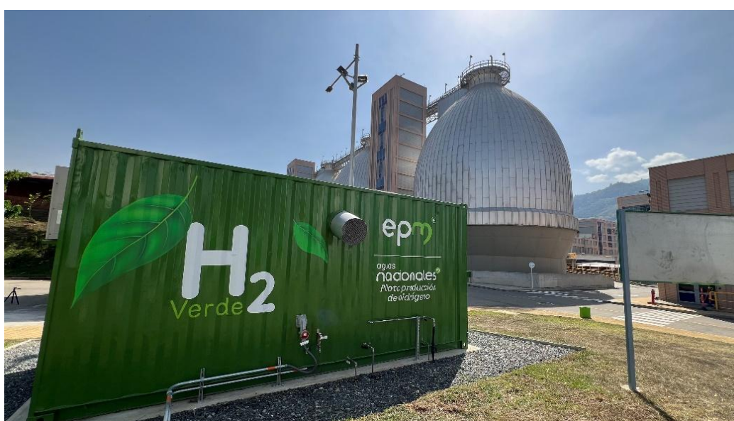
Figure 2-8. Green Hydrogen plant Aguas Claras (EPM, 2023)
